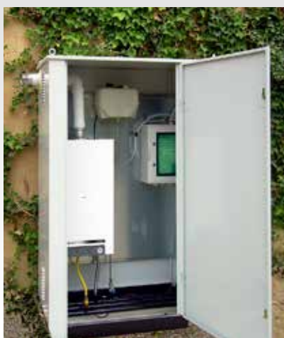
Vapotherm boiler unit Centrale termica Vapotherm
