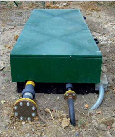
External view with underground tank Vista esterna con serbatoio interrato
